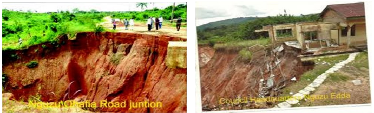
Figure 5: Typical erosion sites in Nguzu Ohafia/Edda, Ebonyi state (Source: News agency of Nigeria, 2011)
